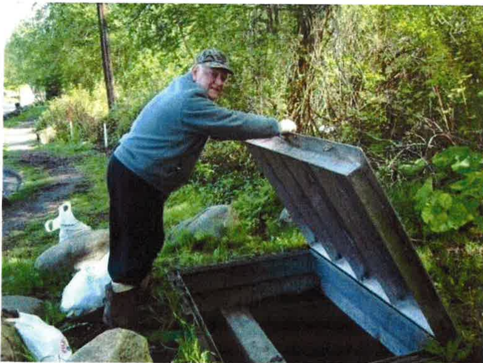
Photo 16 An oil – grit separator near Site 1, provides some treatment of road runoff in commercial and industrial area. These structures require periodic maintenance to remove accumulated oil and sediment.
