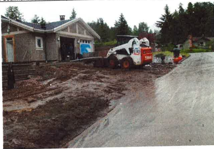
Figure 12: Poor sediment control during landscaping was the major source of TSS and turbidity in June 2008.
