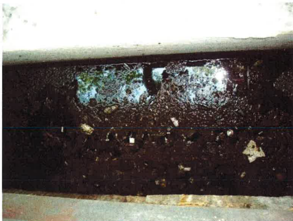
Photo 17 Inside the oil – grit separator.
