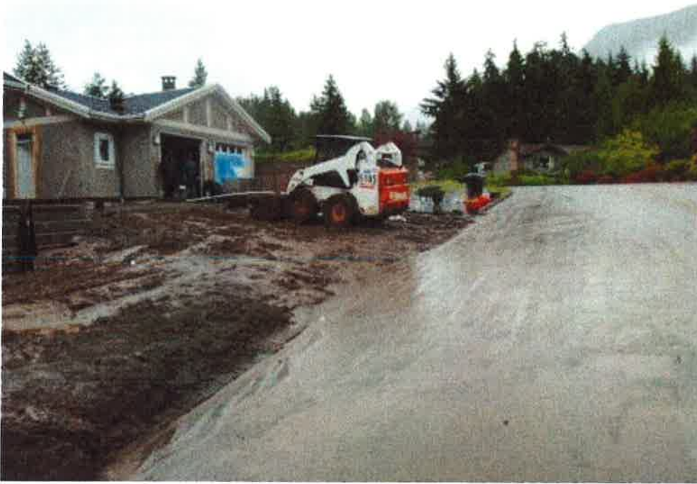
Photo 13 June – this improperly managed landscaping site was unprepared for rain and was the source of highly turbid water – 5 km of stream ran brown for several hours (total suspended solids up to 134 mg/L, turbidity of 55 NTU, well above water quality guidelines). Silt damages fish gills and clogs stream substrates.
