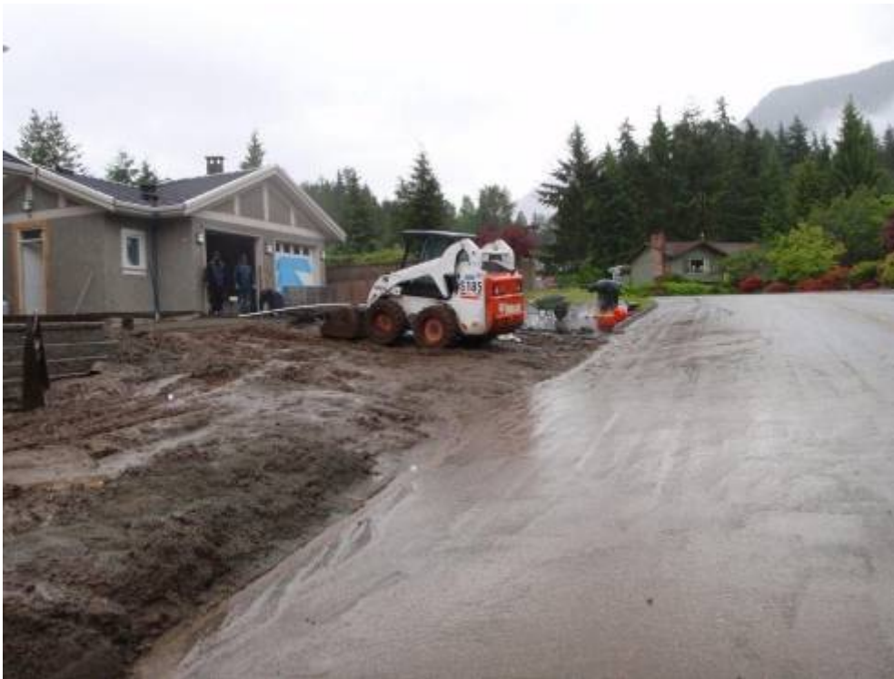
Photo 13 June – this improperly managed landscaping site was unprepared for rain and was the source of highly turbid water – 5 km of stream ran brown for several hours (total suspended solids up to 134 mg/L, turbidity of 55 NTU, well above water quality guidelines). Silt damages fish gills and clogs stream substrates.
