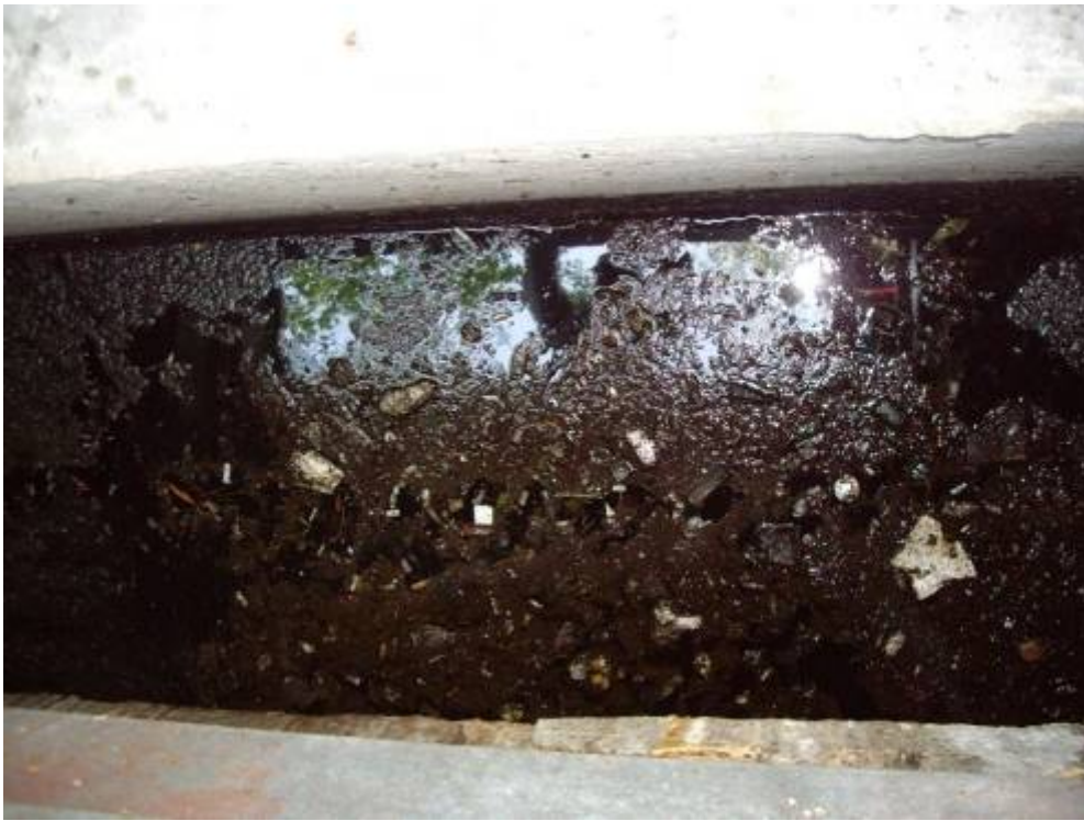
Photo 17 Inside the oil – grit separator.
