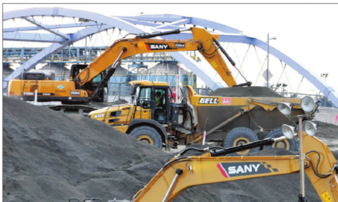
The site on McKean Avenue, in this image from January, is preloaded with sand and gravel to replicate the weight of the future facility before construction of the foundation.
